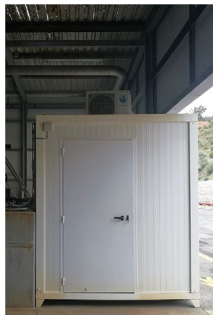
Container on the plant premises containing measurement instrumentation and control unit.
